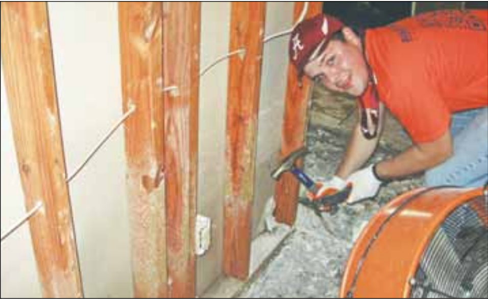
Justin Miller works inside a flood-damaged home in LaPlace, La. Miller survived the 2011 tornado that destroyed a Church of Christ building in Tuscaloosa, Ala., by hiding in a closet.
