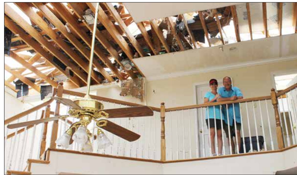
Sunlight shines through the ceiling of Jeff and Jamie Dugger's tornado-damaged home in Cleburne, Texas. The longtime members of the Westhill Church of Christ hid behind kitchen cabinets during the storm.
